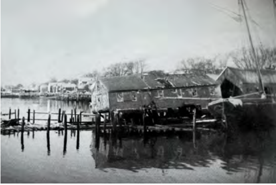
A damaged Union Wharf in Provincetown which was built in 1830-31 is seen here across from Paine's Wharf. Both images are from the collection of Pilgrim Monument and Provincetown Museum.
